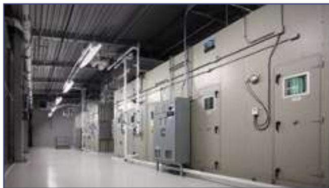
Our processing facility features a one to one ratio of clean rooms to air handling systems
