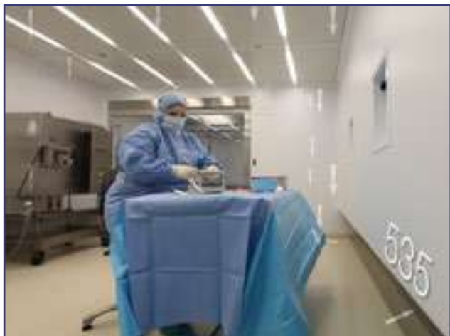
The laminar air flow moves from ceiling to floor and recycles clean air 535 times an hour
